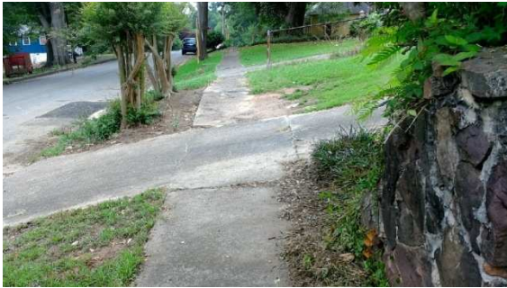
FIGURE 2: NON-COMPLIANT SIDEWALK (DUE TO VERTICAL DISCONTINUITIES AND CROSS SLOPES EXCEEDING 2%, ESPECIALLY AT DRIVEWAY)
