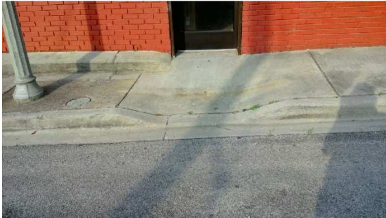
FIGURE 4: NON-COMPLIANT CURB RAMP (DUE TO EXCESSIVE SLOPES, LACK OF DETECTABLE WARNING SURFACE, AND LACK OF TURNING AREA)
