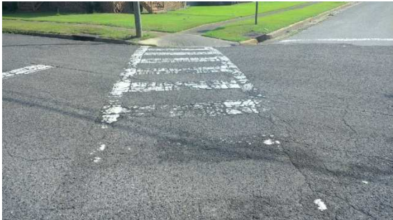
FIGURE 6: NON-COMPLIANT CROSS WALK (DUE TO EXCESSIVE CROSS SLOPES, NEEDS RE-STRIPING IN ORDER TO CONFORM TO CURRENT MUTCD STANDARDS)
