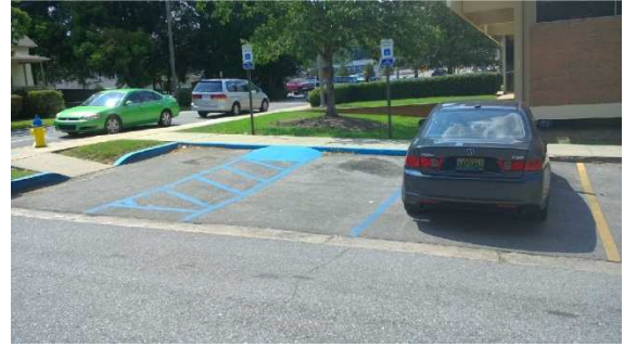
FIGURE 8: NON-COMPLIANT ON-STREET PARKING AREA (DUE TO SLOPES IN EXCESS OF 2% AND LACK OF 8' ACCESS AISLE)
